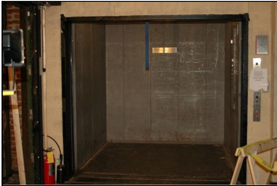
STAGE LEFT FREIGHT ELEVATOR
