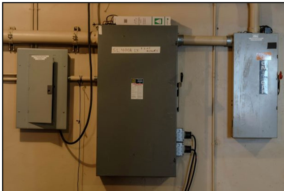
POWER STAGE LEFT PROP ROOM
