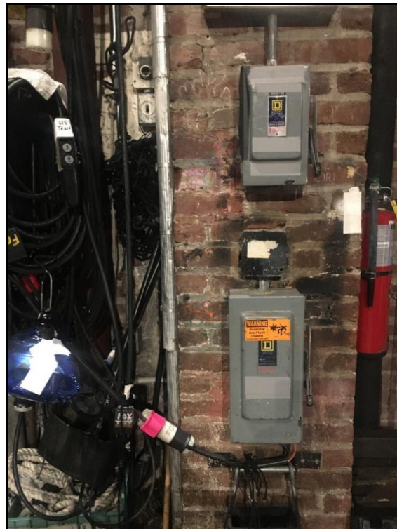
POWER DISCONNECT UP STAGE RIGHT (USR)
